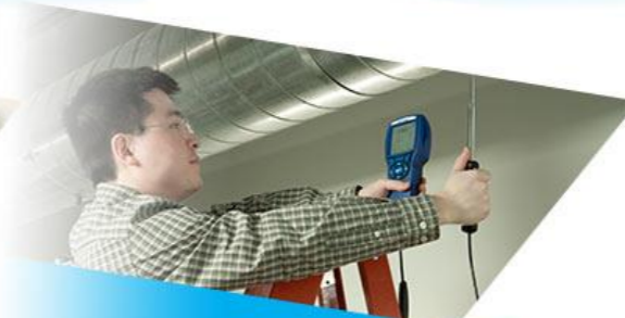
VENTILATION TEST & BALANCE
